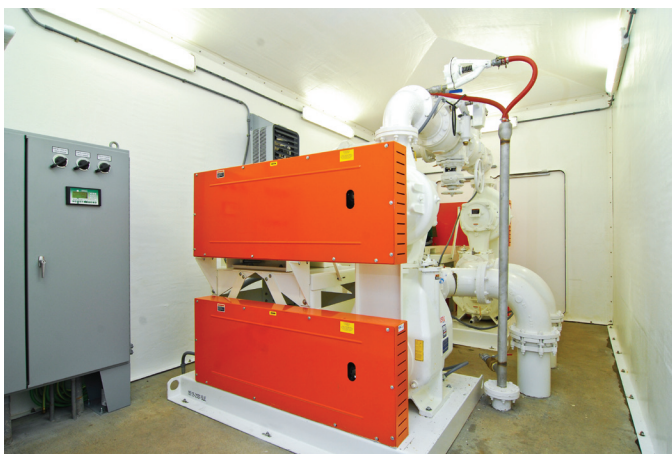
View of a complete set of Ultra-V pumps from the belt drive side. Photos courtesy of Stephen Vitosky.
